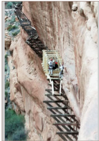
Workers guides work to restore a section of the Hanging Flume in this 2012 picture. The structure — which uses original 120-year-old supports — sits 100 feet above the San Miguel River west of Uravan. Photo special to the Sentinel.
